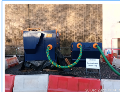
Contaminated waste disposal
